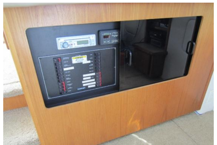
AC/DC electrical panel, stereo & inverter control panel
