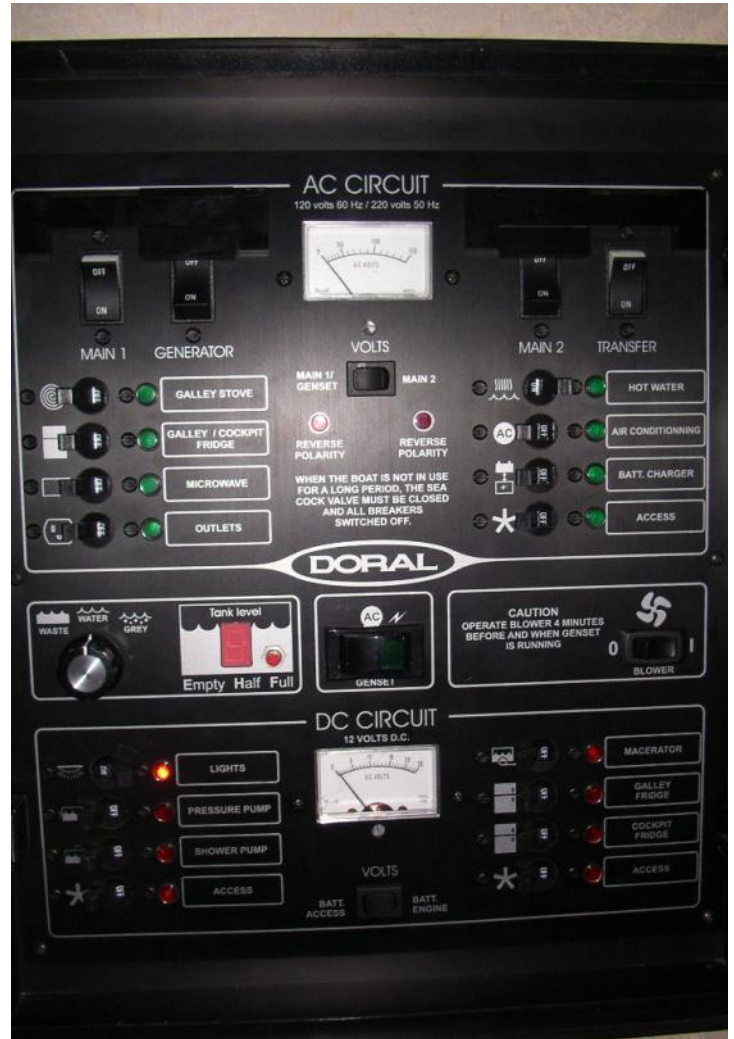
Ship's electrical panel/breakers
